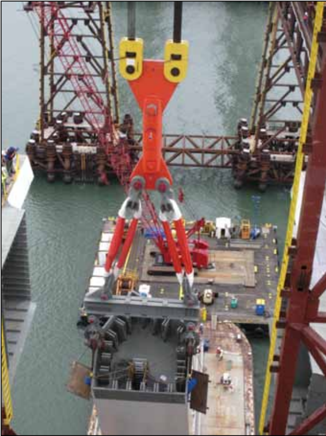
McKissick® 1250 metric ton Swivel and Hangers along with Crosby® 600 metric ton "Wide Body" Shackles lifting 1200 metric ton Bay Bridge Tower.
