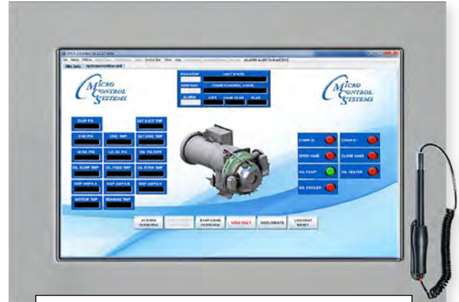
COMPRESSOR OVERVIEW SCREEN
