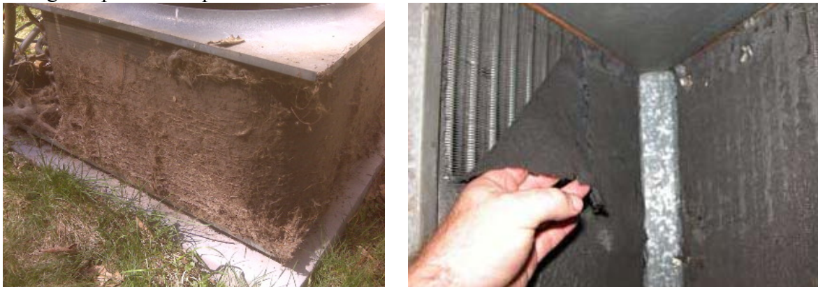
Figure 11. Examples of condenser and evaporator coil fouling.
