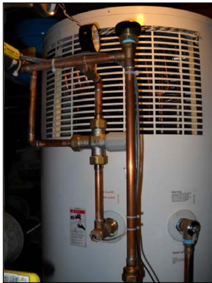
Figure 14. Heat pump water heater with mixing valve
