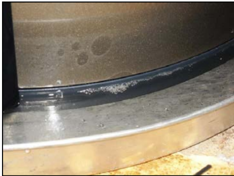
Figure 10. Condensate problems from improper installation
