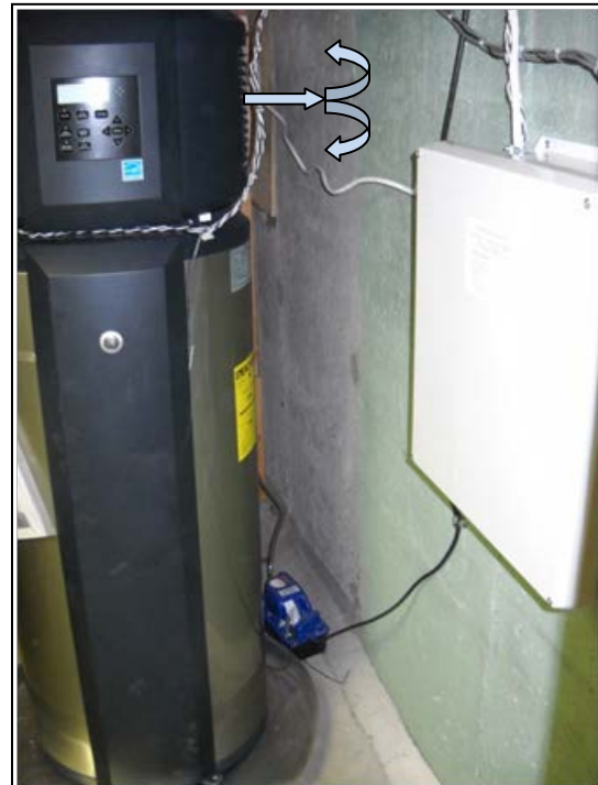
Figure 8. Improper HPWH with air discharge facing wall
