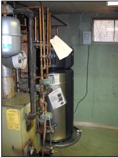
Figure 9. HPWH installed in boiler room
