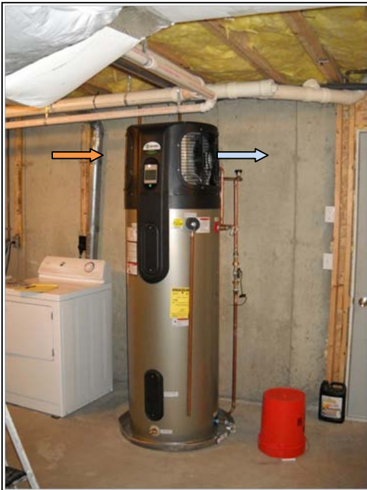
Figure 7. HPWH installed with adequate clearances
