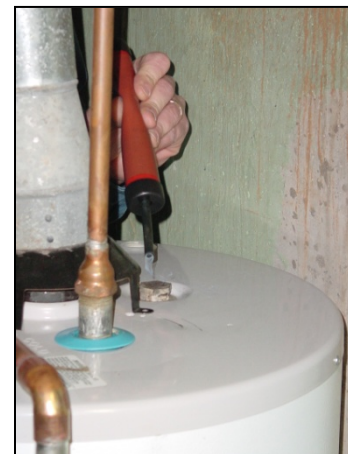
Figure 22. Spillage testing of an atmospherically vented, natural gas water heater
