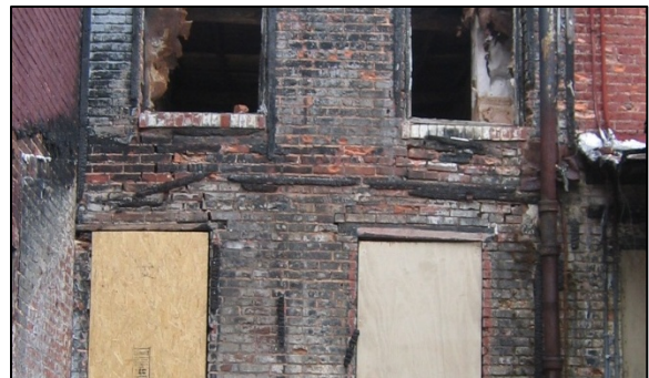
Figure 7. Heavily deteriorated brick wall
