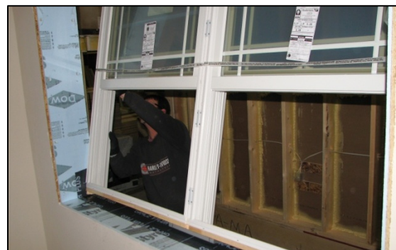
Figure 19. Installing a window after installing insulation and flashing. XPS insulation was placed between the window buck and the interior jamb extension (not yet installed) of this modular home.
