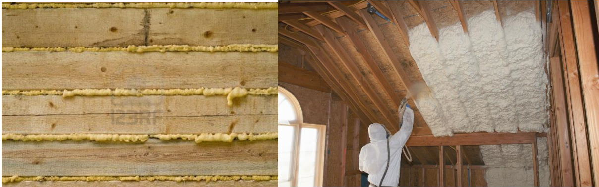
Figure 2.19 Left: PUR injected on site for sealing wooden beams. Right: Spraying PUR foam for thermal insulation in a frame wood roof.
