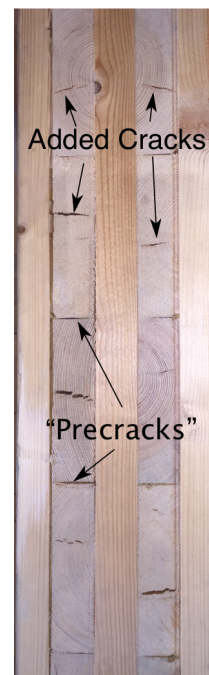
Figure 1: Typical CLT has “precracks” (initial non-glued edges) and “added cracks” induced by environment.
