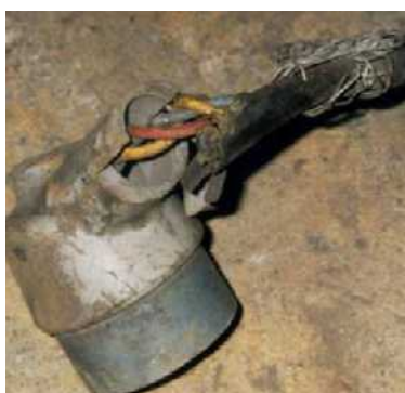
Damaged cable grip
