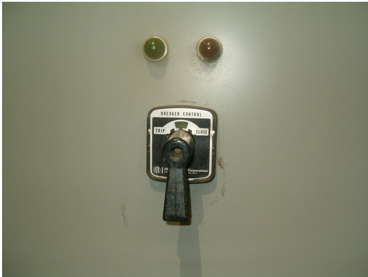
FIGURE 3-1 Cubicle breaker control switch
