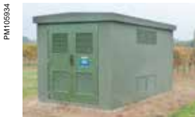
Fig G Example of HV/LV prefabricated substation with 1250 kVA liquid filled transformer, 19kW of losses before EU regulation change
