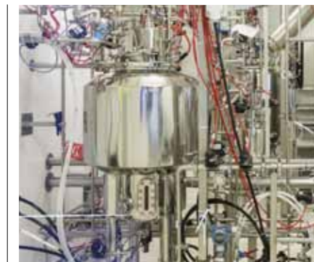
Nested in the mountains of Switzerland TRB Vouvry's plant general view.
