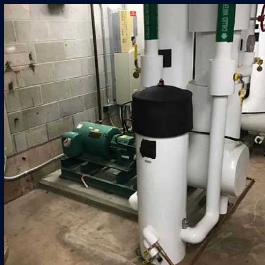
Gampel Chilled Water Pump
