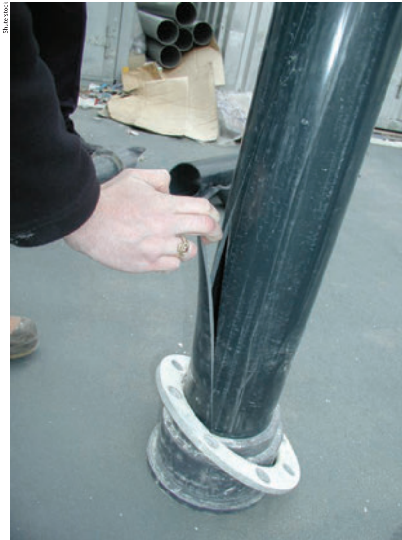
A number of pipe-fitting failures can be attributed to poor installation
