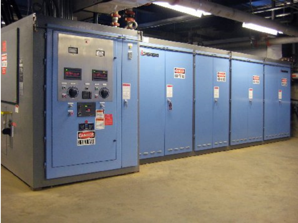
Controls for the induction furnaces
