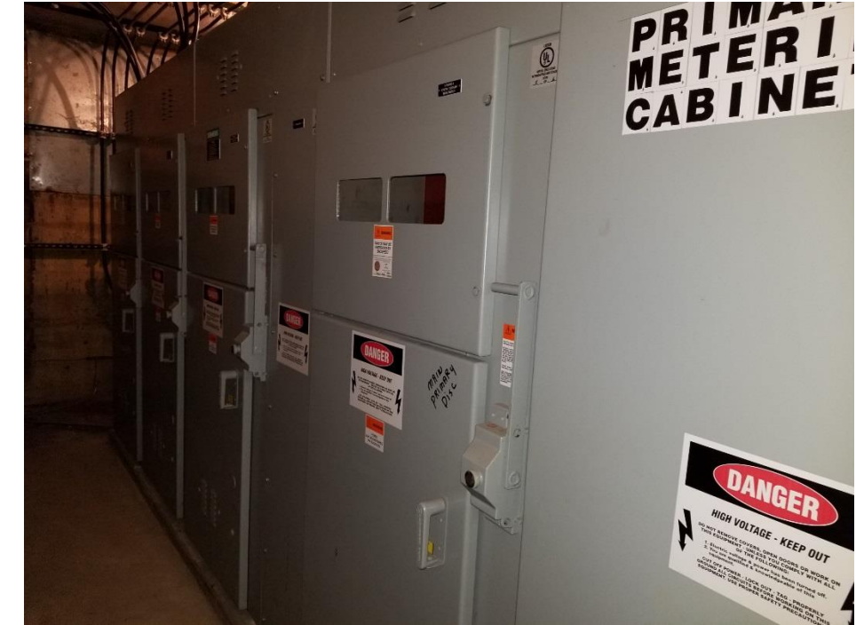
ComEd Vault Switchgear
