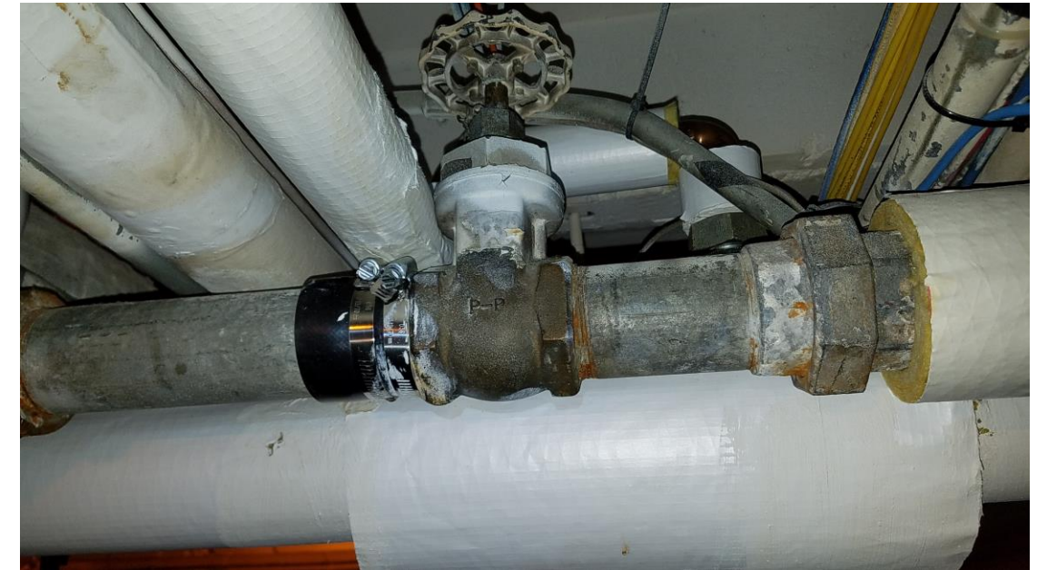
Sample of Failed Existing Galvanized Piping
