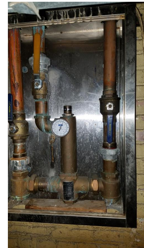
Master Mixing Valve to be Replaced
