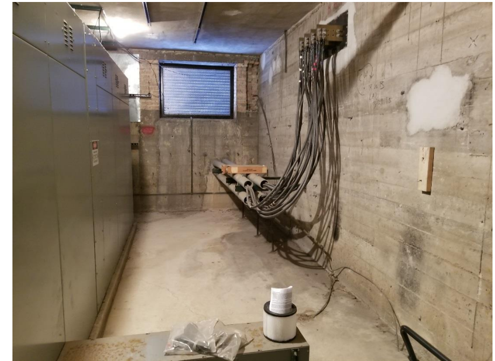
Secondary Cables to Basement Electrical Room
