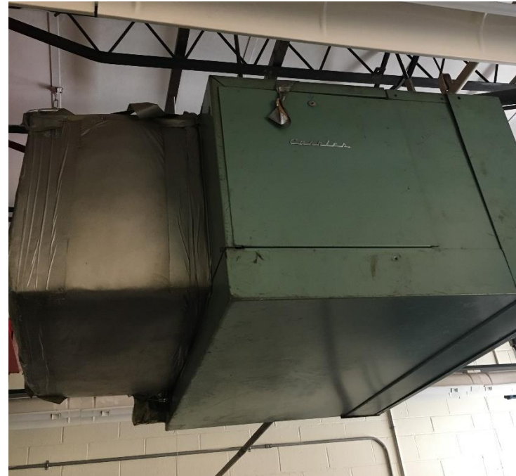
1. Copy Room AHU
