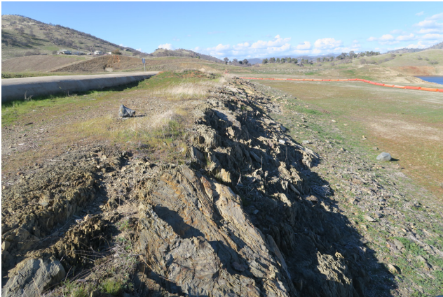
Ungated spillway lip at left, fractured rock below
