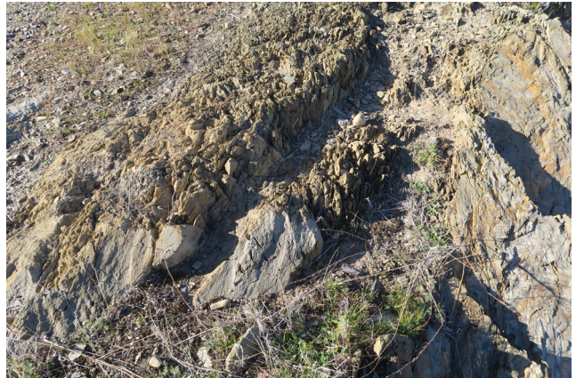
Closeup of fractured rock below ungated spillway
