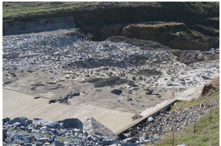
2018 view. Note rough concrete pour next to concrete apron slabs and shotcrete stabilization downstream
