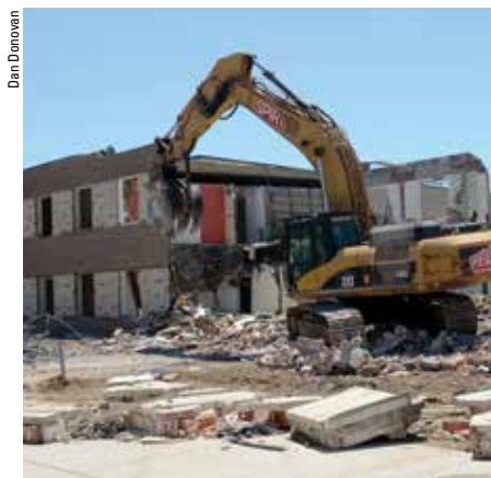
DEMOLITION: Workers level Duchesne Hall, a residence hall built in 1960. A key feature of Myrtle E. and Earl E. Walker Hall is that it incorporates numerous energy conservation and green construction technologies.
