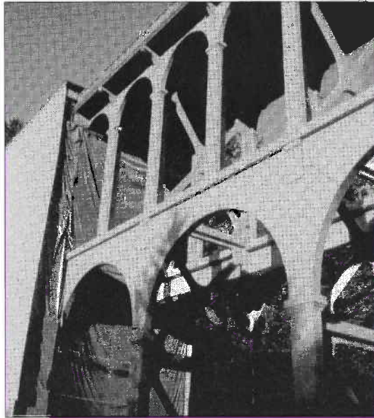
Cape Creek Bridge, Oregon. The first complete structure to use zinc metallizing in a cathodic protection application.
