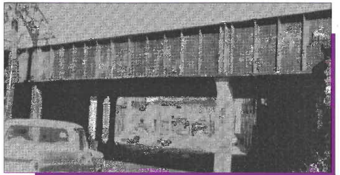
Ridge Avenue Bridge in Philadelphia, Pennsylvania Zinc Metallized in 1930's. To date this bridge is still essentially corrosion free.
