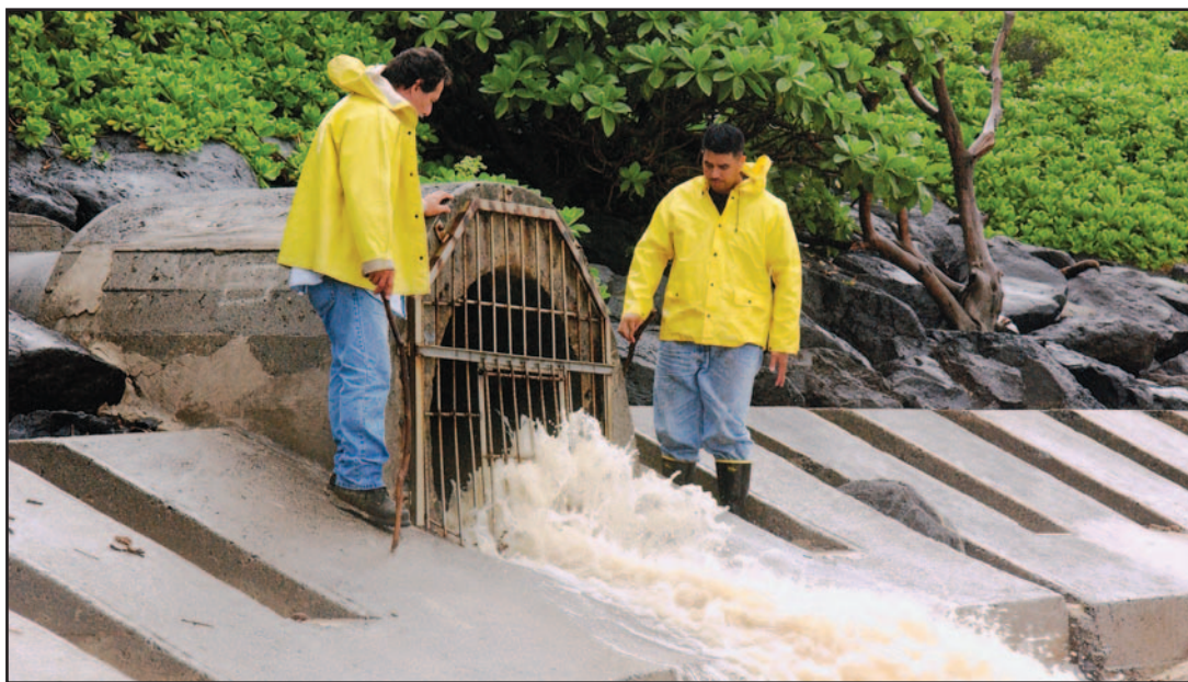
Andrew Baldauf (left), 51, and Kevin Aipoalani, 28, civil service workers with Base Facilities and Maintenance Division, clean out the Pond Road storm drain at North Beach, here.
