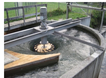
Figure 2 – Vortex Power Generation 4
