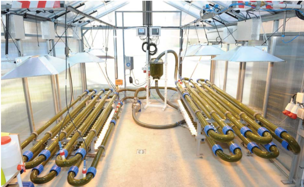
Figure 18 Photobioreactor at Duernrohr power station (Kinger, 2015)
