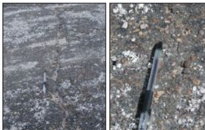
Crack in moist-cured section.
