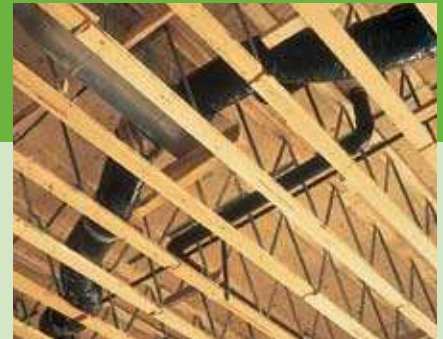
The open-web structure of these trusses allows easy placement of plumbing and ductwork, as shown in this retail shopping mall.
