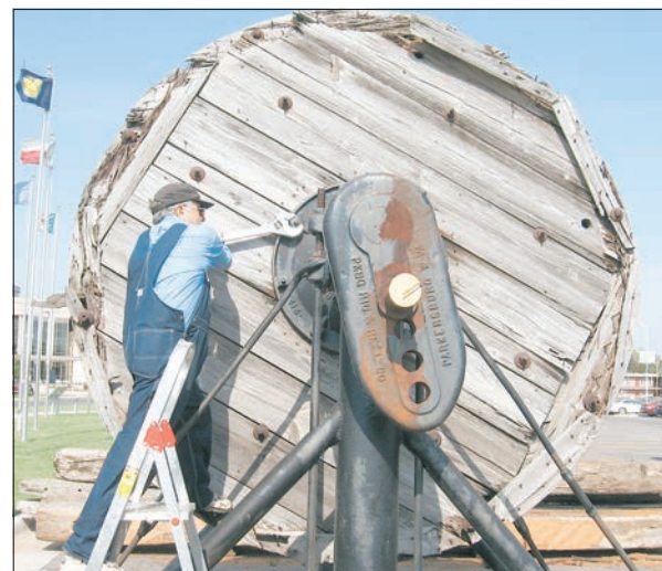
Repairing the band wheel to add to the power plant (Everett photo).
