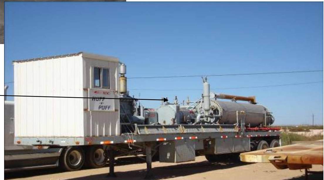
Pump and flow control equipment
