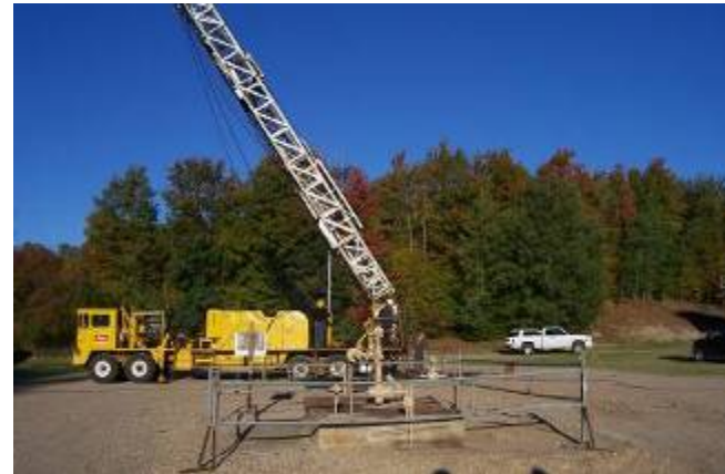
Monitoring Well (about 500 feet from injection well)
