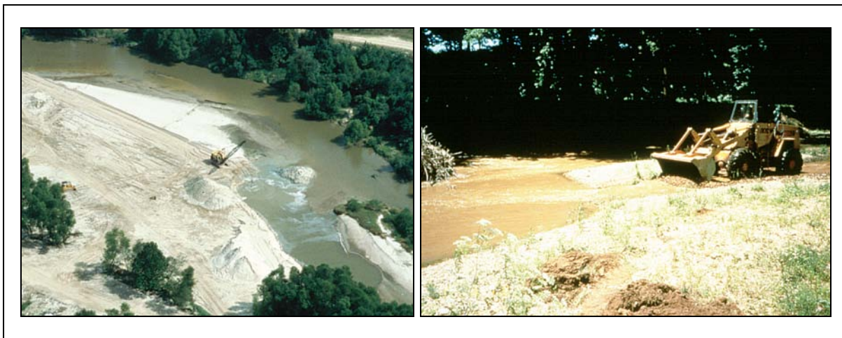
Figure 3.14: Excavating Sand and Gravel from Stream Channels Using Conventional Earth Moving Equipment (Langer, 2003)
