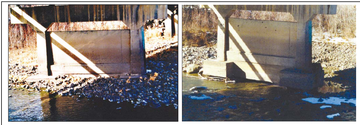
Figure 2.8: The left photograph shows a bridge abutment in 1992. The right photograph shows the same abutment during 1995. The bridge scour (erosion of river beds at bridge foundations) is due in part to in-stream mining and in part to channelisation of the river (Langer, 2003)
