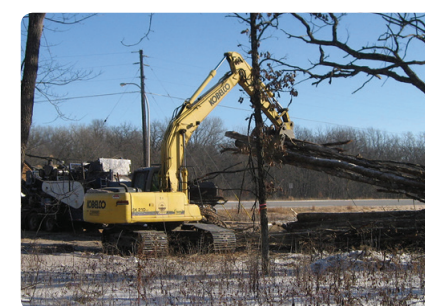
Downed trees and waste wood were taken from Frontenac State Park to generate energy.
