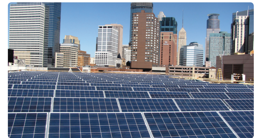
More than 2,600 solar panels sit atop the Minneapolis Convention Center and help directly power the facility. (Photo Credit: Minneapolis Convention Center)
