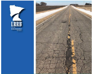
A Guide to Successfully Convert Severely Distressed Paved Roads to Engineered Unpaved Roads
