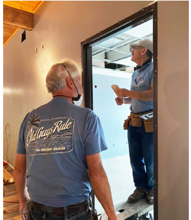
Pastor Larry Creamer and Tom Wokosin of Valley Baptist Church in Appleton, Wis., install a door frame in the new addition at Journey Church of Amery, Wis. Charles Dunning led the Builders for Christ volunteer building team of Valley Baptist Church in the project as 17 volunteers participated Aug. 16-21 and 16 volunteers participated Aug. 23-28. The 2,300 square foot addition increased Journey Church's worship seating by 50 percent to 250, increased their greeting space, and added two classrooms, large restrooms and a nursery. "We were primarily completing the interior finishing work," Dunning said, adding that one couple worked outside completing the exterior fascia and soffits. "Inside we installed eight suspended ceilings, 17 doors and door frames, all of the main level floor covering, partitions in the restrooms and trim on the windows." Derek Downs is pastor of Journey Church.
