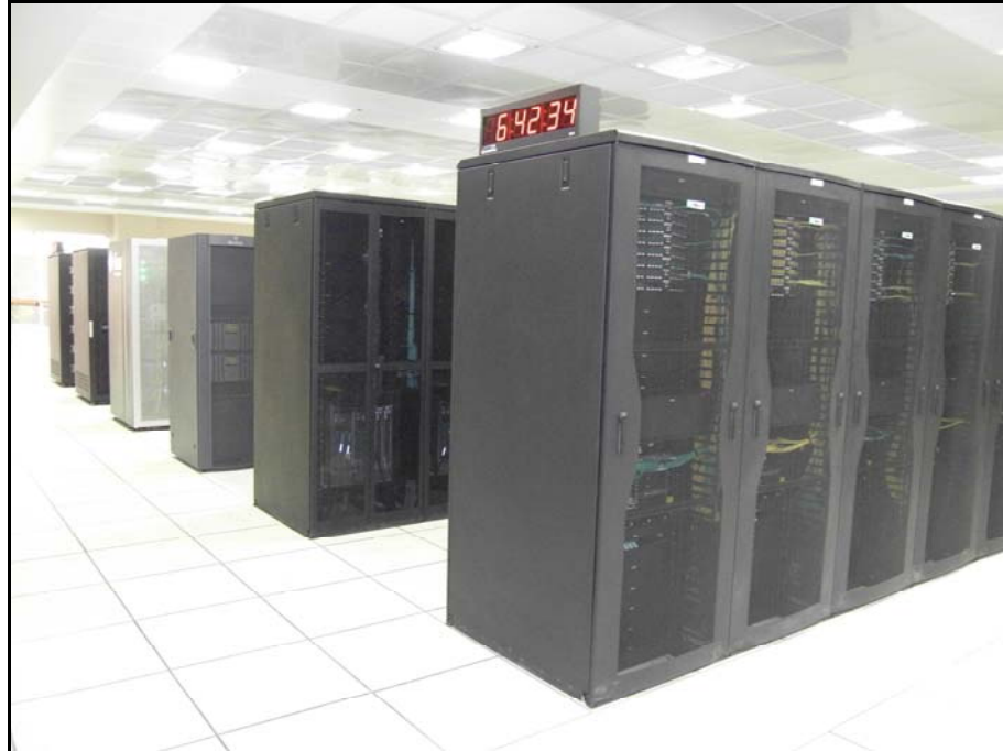
Fig. 1. Indian Space Science Data Center
