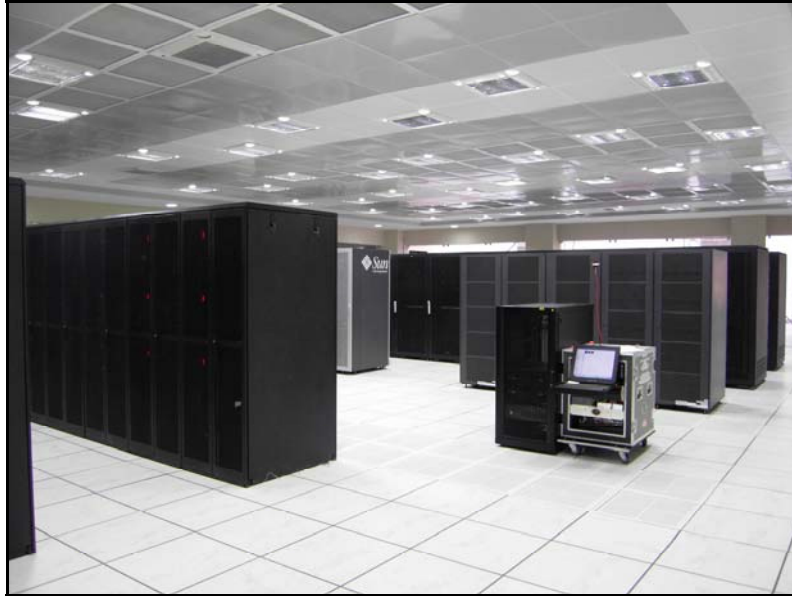
Fig. 2. Indian Space Science Data Center
