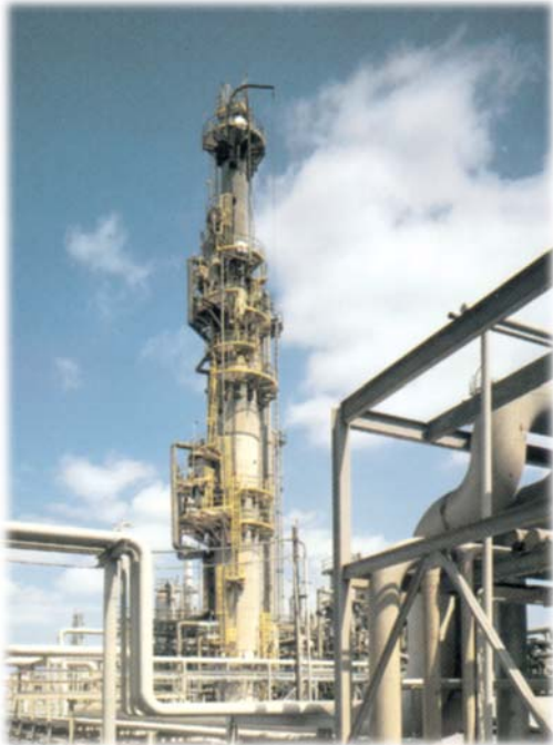
Fractionation tower in a major USA refinery.
