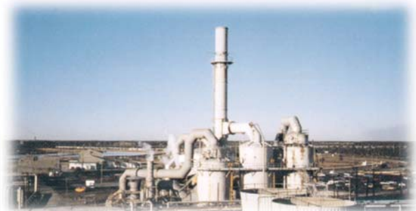
Sulfuric acid plant using KOCH-OTTO YORK® mist elimination technology.
