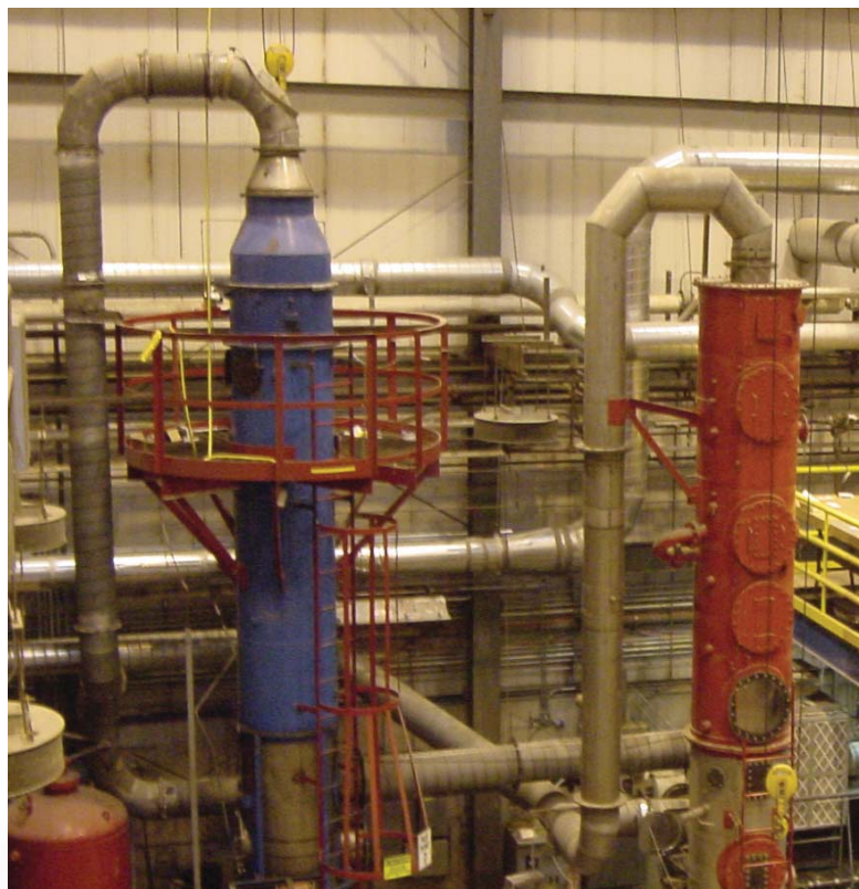
These two test towers are devoted to the research and development of new FLEXIFIBER® mist eliminator designs. The latest BD-LdP low pressure drop designs came from test work performed in these towers.
