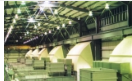
Air intake area at the Lumut Power Plant Kawasan penyedutan udara di Loji Janakuasa Lumut
