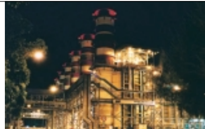
Night vision of the Lumut Power Plant Pemandangan di waktu malam Loji Janakuasa Lumut
