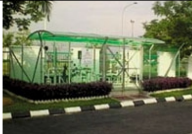
Regulating station Stesen pembahagian
