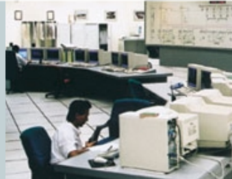
Main control room of the Lumut Power Plant
