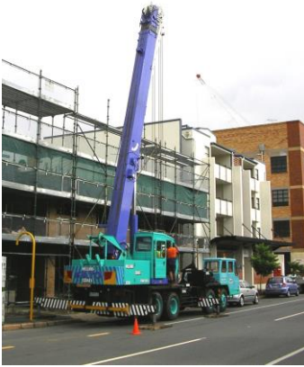
Figure 2 – Hazard striping on a mobile crane
