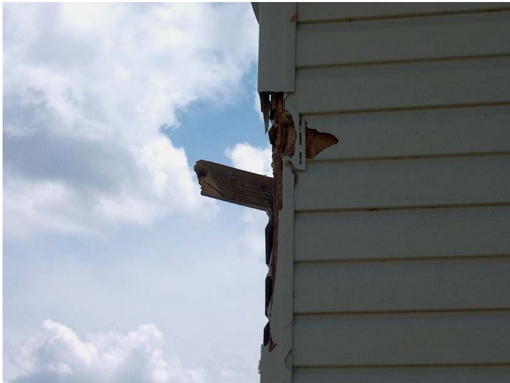
Figure 6.32: Damaged Corner Part of the Home
