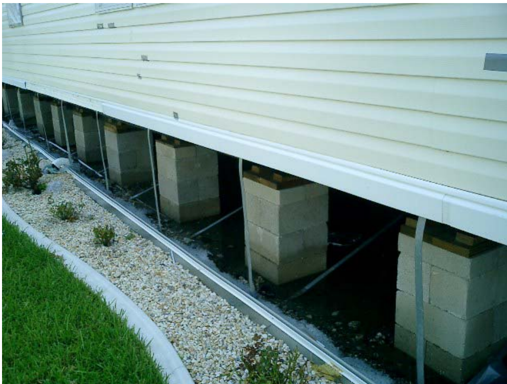
Figure 6.24: Manufactured Home Installed in Accordance with Florida Installation Law with Anchors at about 5 ft. on Center.
