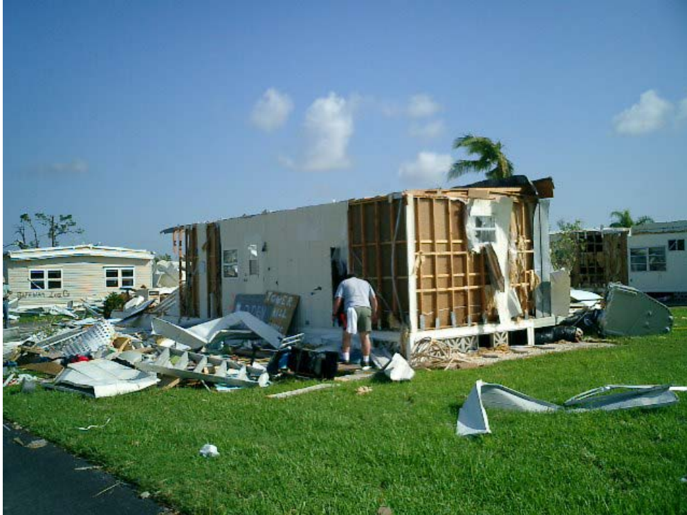
Figure 6.15: Destroyed Manufactured Home Built Prior to 1976
