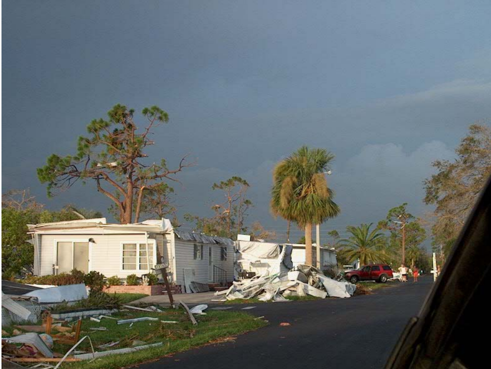
Figure 6.17: Failure of Roof System
