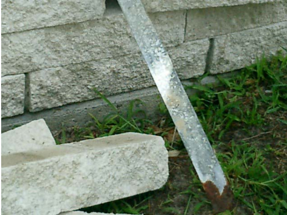
Figure 6.31: Corroded Ground Anchor Strap
