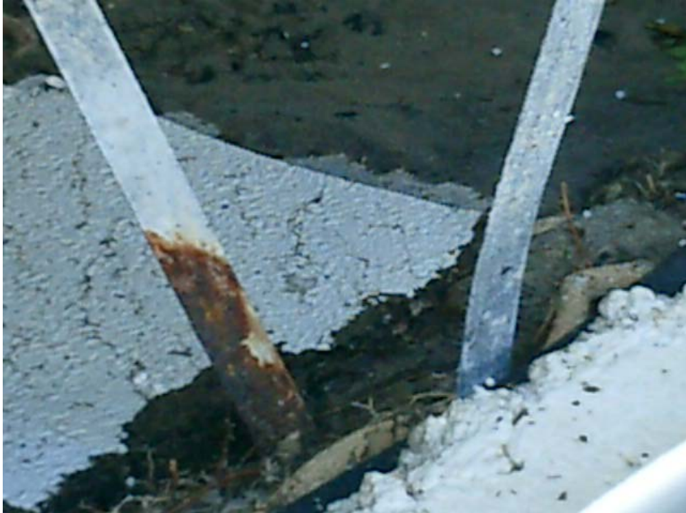
Figure 6.27: Corroded Ground Anchor Strap
