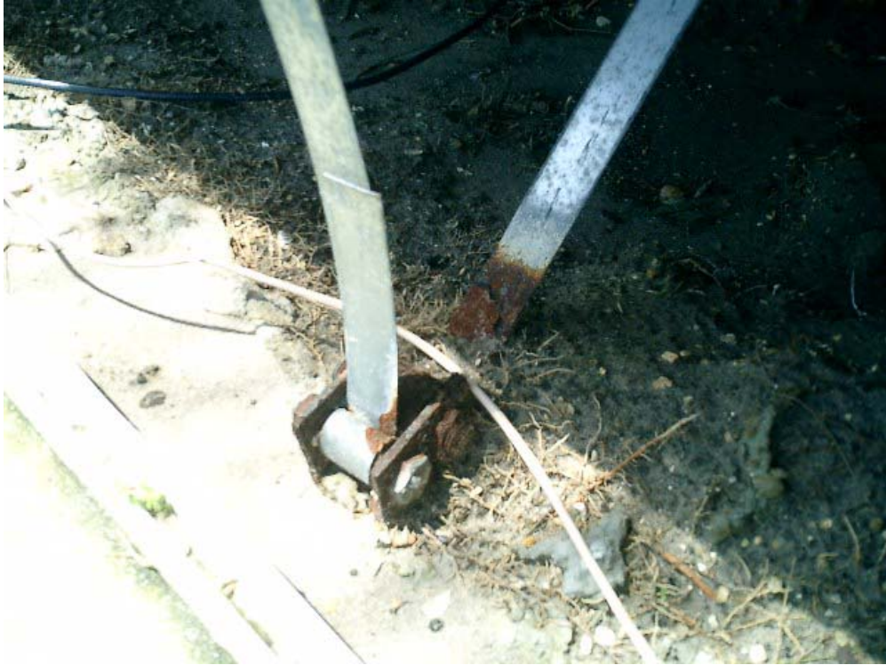
Figure 6.29: Corroded Ground Anchor Strap
