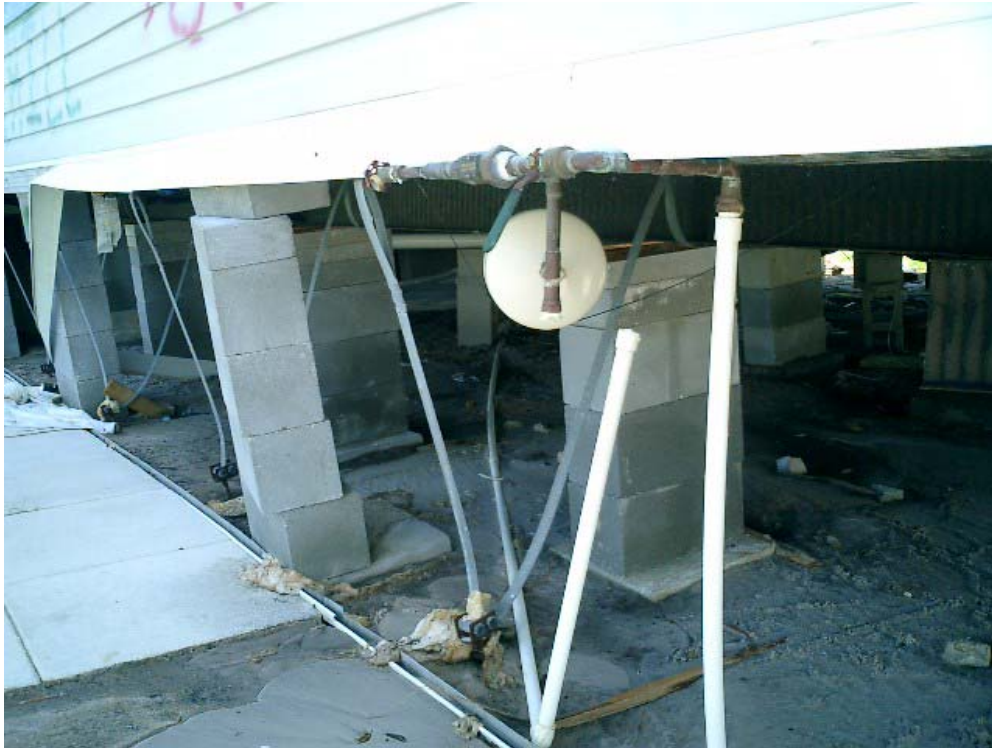
Figure 6.23: Manufactured Home Slightly Shifted from its Foundation
