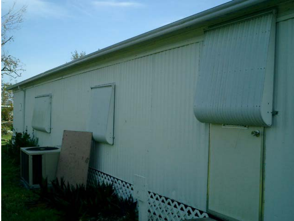
Figure 6.21: Manufactured Home with Shutters Survived Hurricane Wind Forces
