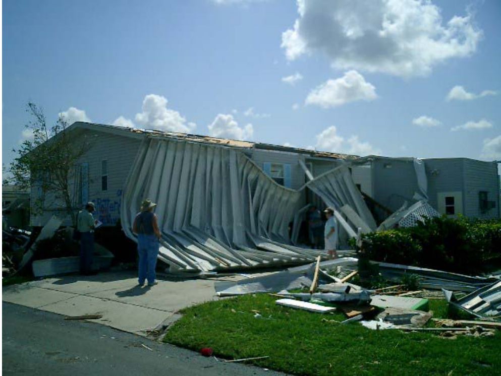
Figure 6.5: Destroyed Add-On Construction
