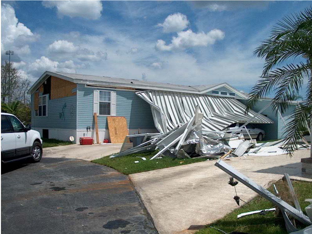
Figure 6.4: Destroyed Add-On Construction
