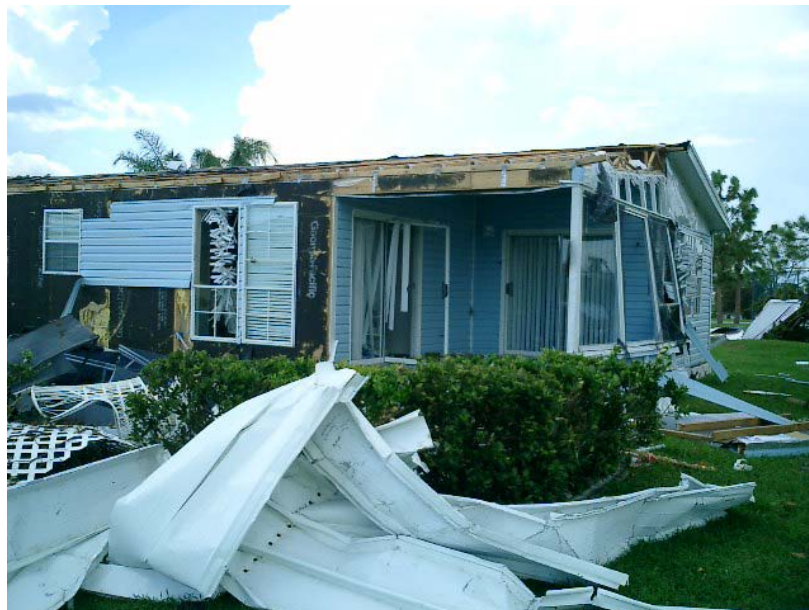
Figure 4.1: An Example of Level 3 Roof System and Level 2 Wall System Damage [Note: In this case, the roof rating was primarily associated with extensive roof sheathing loss; the wall rating was based on some localized structural damage to sheathing in addition to extensive siding damage, even though the walls were essentially structurally intact.]
