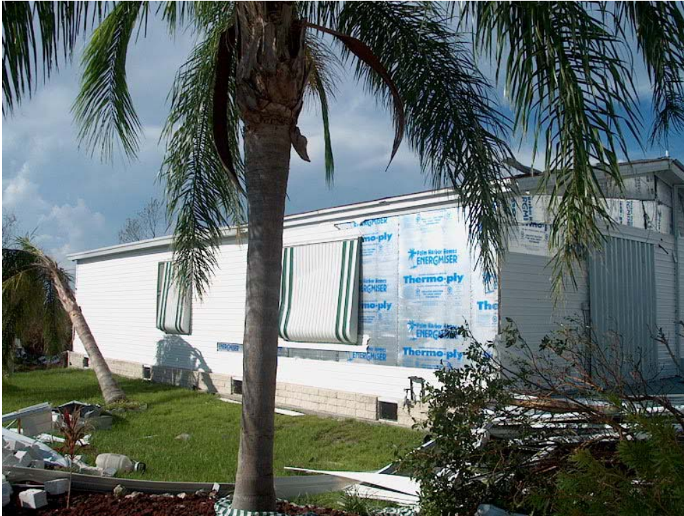
Figure 6.7: Damaged Sidewall and Endwall Siding
