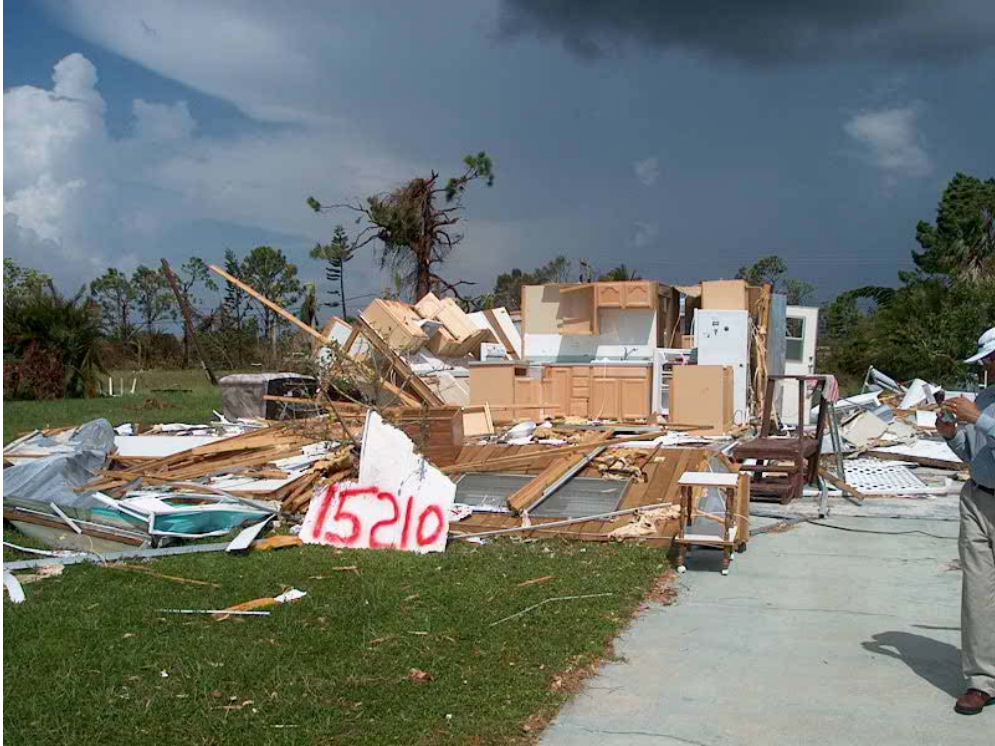
Figure 6.9: Destroyed Manufactured Home
