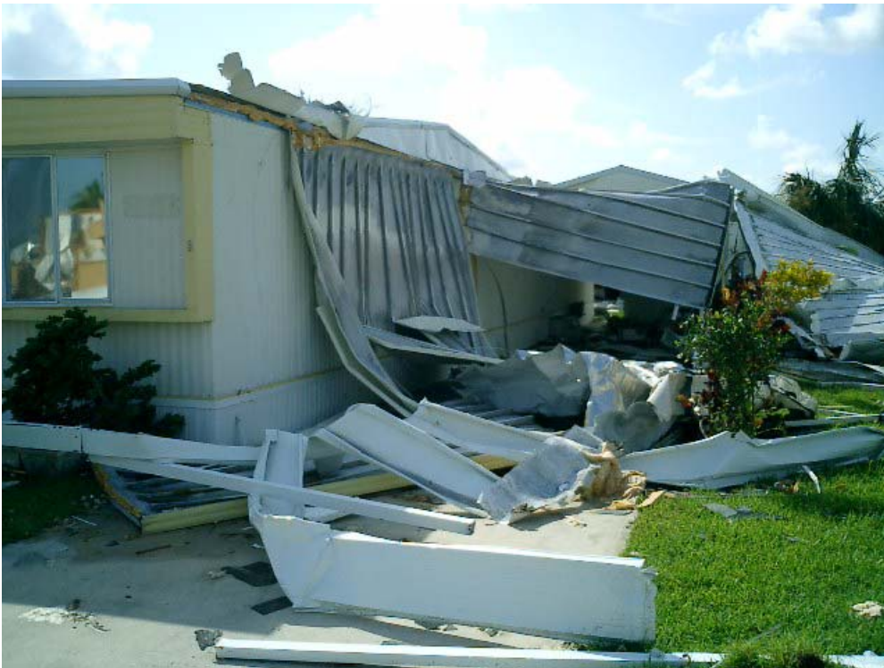
Figure 6.2: Destroyed Add-On Construction
