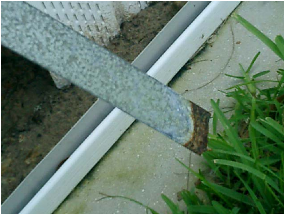
Figure 6.28: Corroded Ground Anchor Strap
