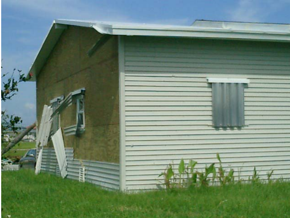
Figure 6.33: Damaged Endwall Siding
