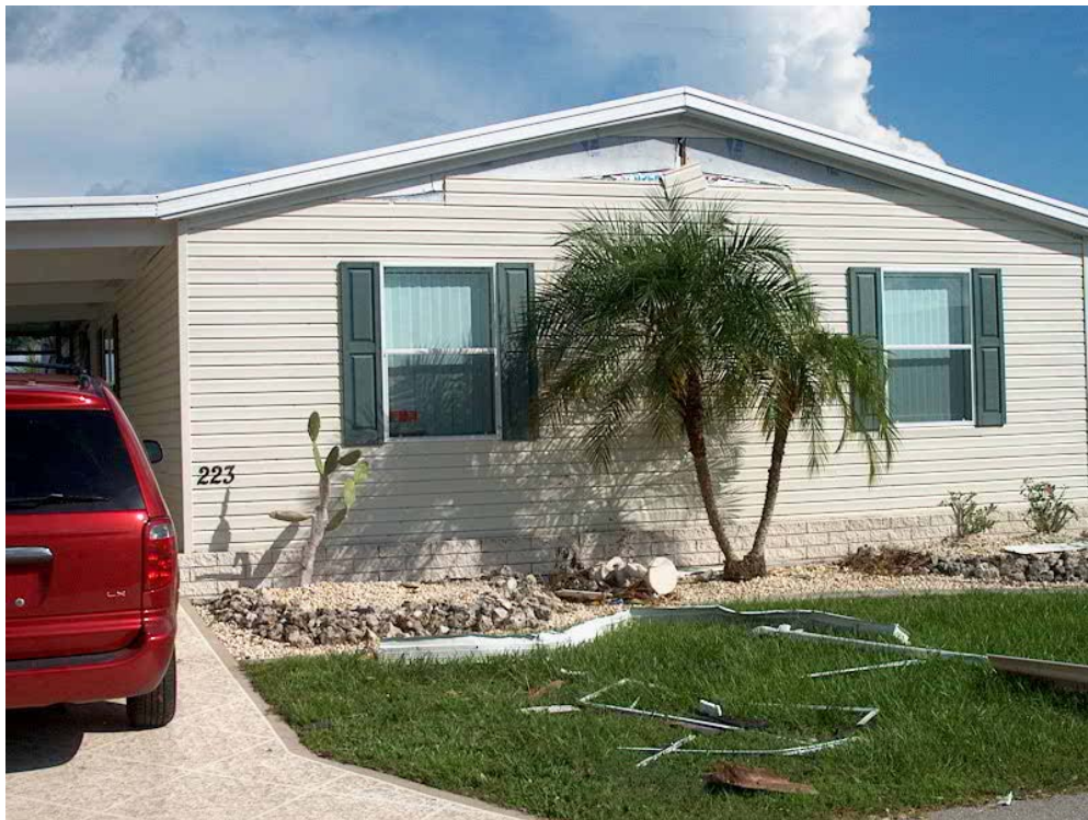
Figure 6.36: Damaged Endwall Siding
