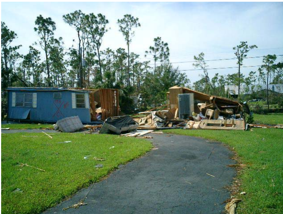
Figure 6.14: Destroyed Manufactured Home Built Prior to 1976
