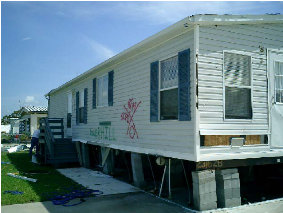
Figure 6.22: Manufactured Home Slightly Shifted from its Foundation
