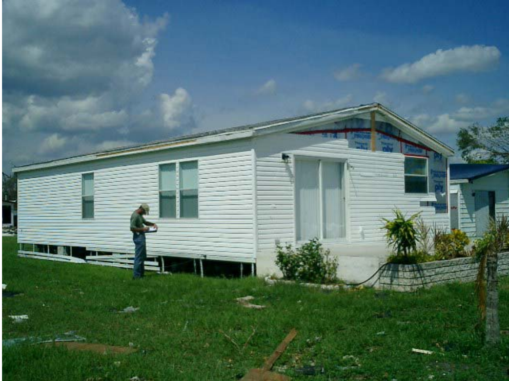
Figure 6.35: Damaged Endwall Siding
