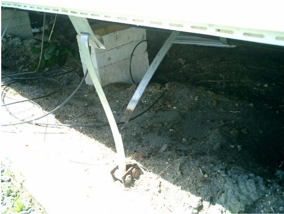
Figure 6.30: Corroded Ground Anchor Strap
