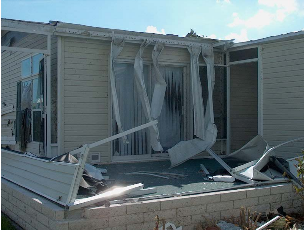
Figure 6.1: Destroyed Add-On Construction
