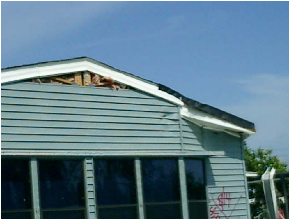
Figure 4.3: An Example of Level 1 Wall System Damage [Note: Damage was limited primarily to wall finishes, i.e. vinyl siding damage]
