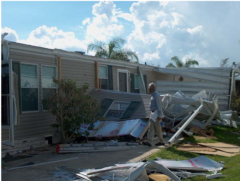
Figure 6.6: Destroyed Add-On Construction
