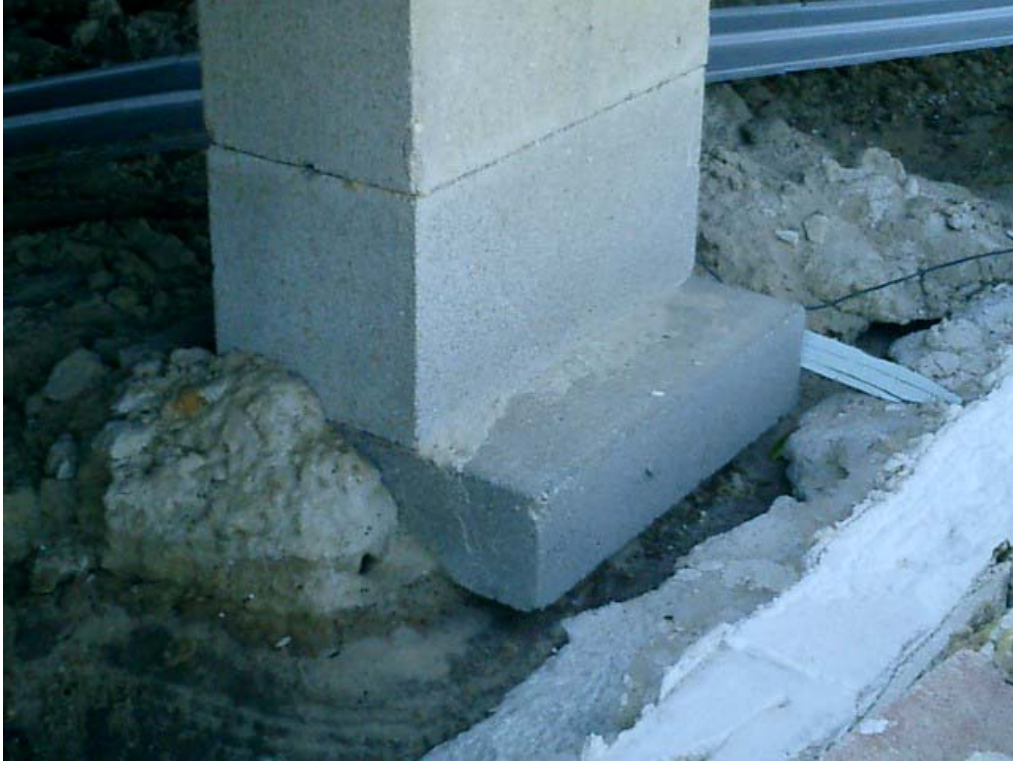
Figure 6.37: Scouring Action of Wind and Rain Water Runoff
