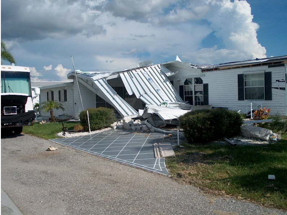
Figure 6.3: Destroyed Add-On Construction
