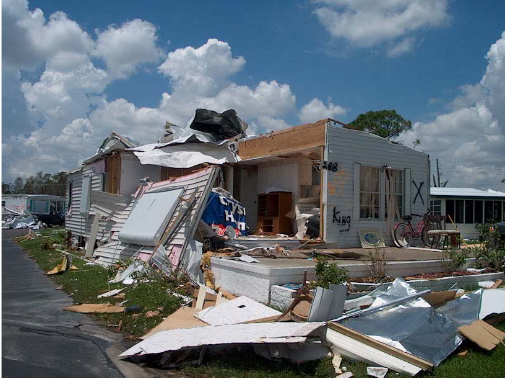
Figure 6.11: Failure of Wall and Roof System
