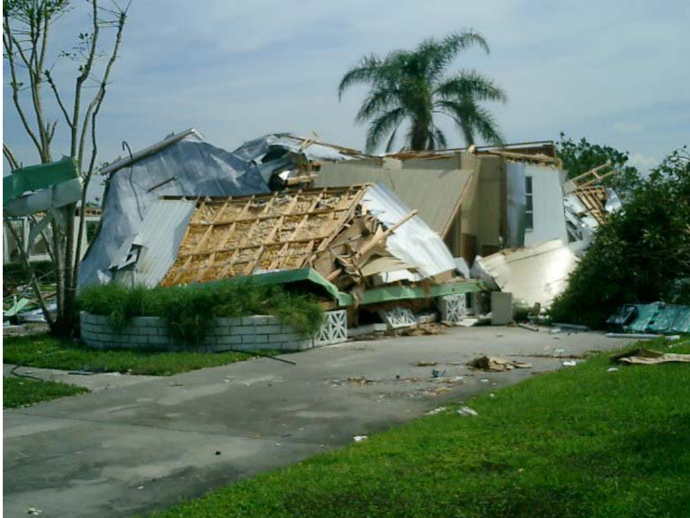
Figure 6.13: Destroyed Manufactured Home Built Prior to 1976
