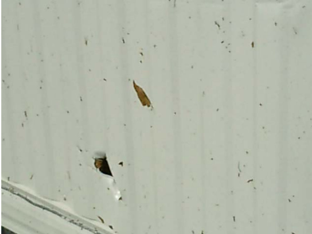
Figure 5.1: An Example of Debris Penetrating a Wall
