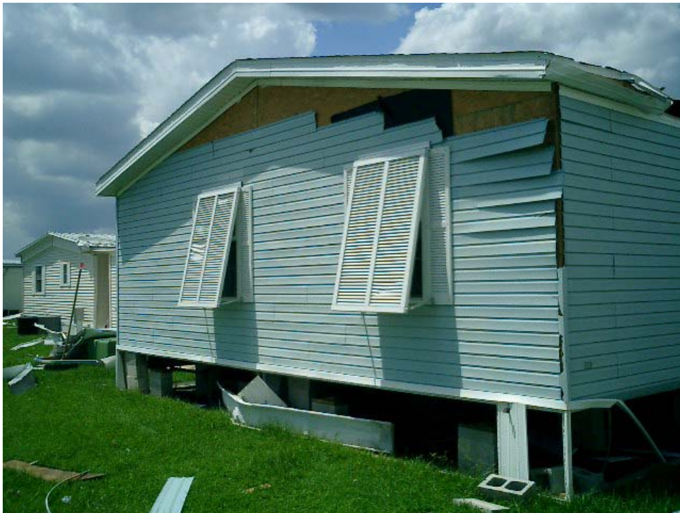
Figure 6.34: Damaged Endwall Siding
