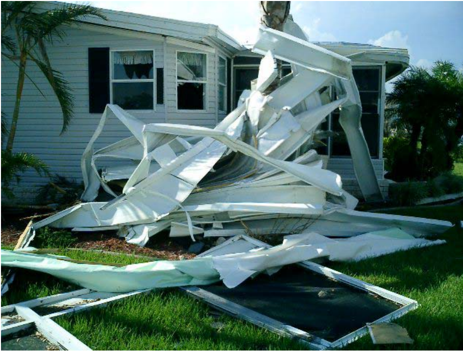
Figure 5.2: An Example of Substantial (Level 3) Add-On Damage
