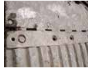
Damaged clamping wedges
