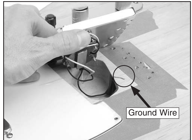
Figure 23. Ground wire above bridge cavity.
