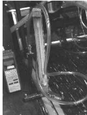
Figure 2-1 Flow meter 2, a variable area flow meter.
