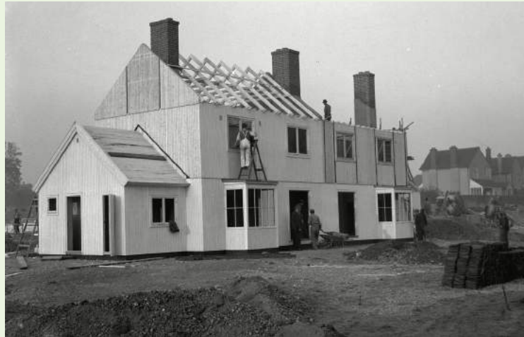
Builders, supervised by Swedish foremen, work to complete the first of six Swedish-made prefabricated timber houses, at Abbots Langley, Hertfordshire, 1945
