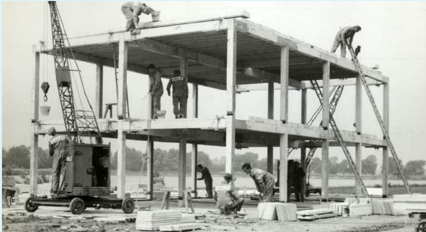
Workmen constructing the precast concrete frame of an Orlit prefabricated house, circa 1945. Seventeen thousand were built from the 1940s to 1950s. Designated defective!
