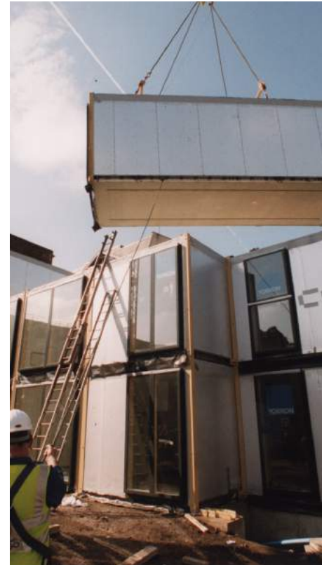
Murray Grove, London, 1999, volumetric construction using light steel frame for dense urban housing
