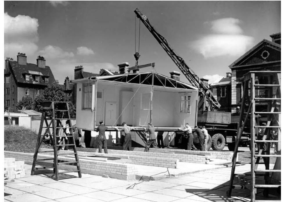
An exhibition prefabricated house under construction in the grounds of the Tate Gallery, London, 1945, showing the first section being swung into position onto the brick base
