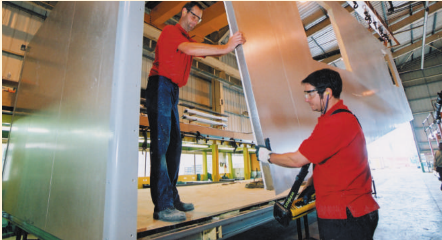
Steel framed room modules are manufactured and fully fitted out in a British factory
