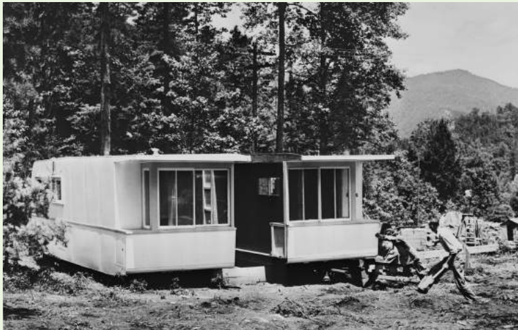
Construction of experimental trailer houses for Tennessee Valley Authority workers in western North Carolina
