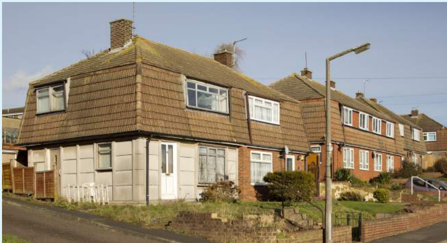
Cornish Unit precast concrete houses, Hoo Peninsula, Medway, Kent. Thirty thousand bungalows, semi-detached and terraced houses were built from 1946 to the 1960s. Designated defective!
