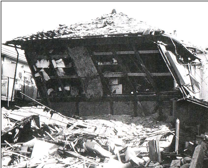
Figure 7: Ductile deformation of a traditional timber house damaged by Kobe earthquake in 1995 (photo: Shigeo Ohira).
