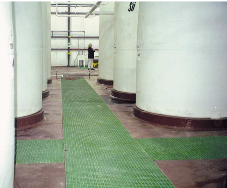
The Exide Battery Plant in Manchester, Iowa installed corrosion resistant DURAGRATE® around its tanks of sulfuric acid.
