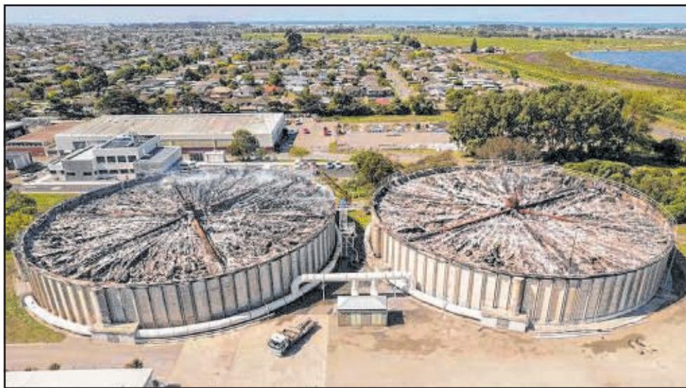
THE BIG STINK: Drone footage shows the extent of the damage to the plant's roof.
