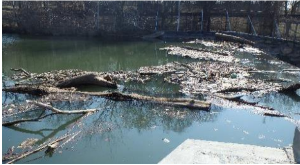
Photo 9: Debris build-up on top of dam
