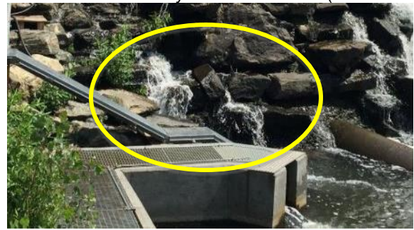
Photo 8: Water leaking from dam (yellow circle)
