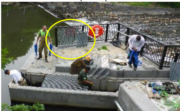
Photo 10: Metal grates placed against the railing (yellow circle)
