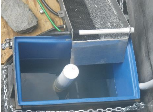
Photo 21: Holding tank with screen attached and location of the upper spray bar
