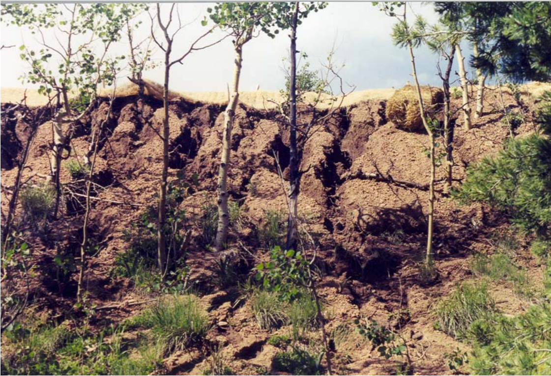
Figure 3. View of fill slope 039FS from the upper silt fence taken on June 30. Note the straw bales lining the top of the slope and in the upper right of the picture.
