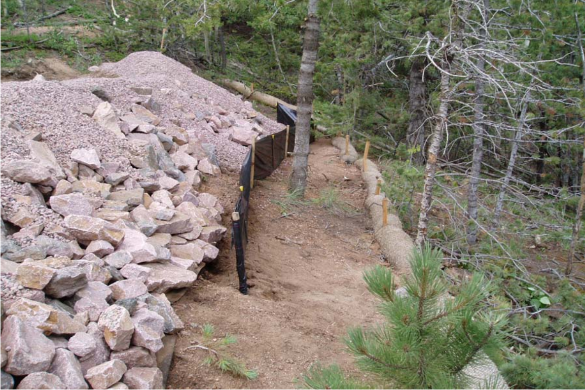
Figure 6. Slope below 152RW after storm on July 29. Note lack of transported material below excelsior logs.
