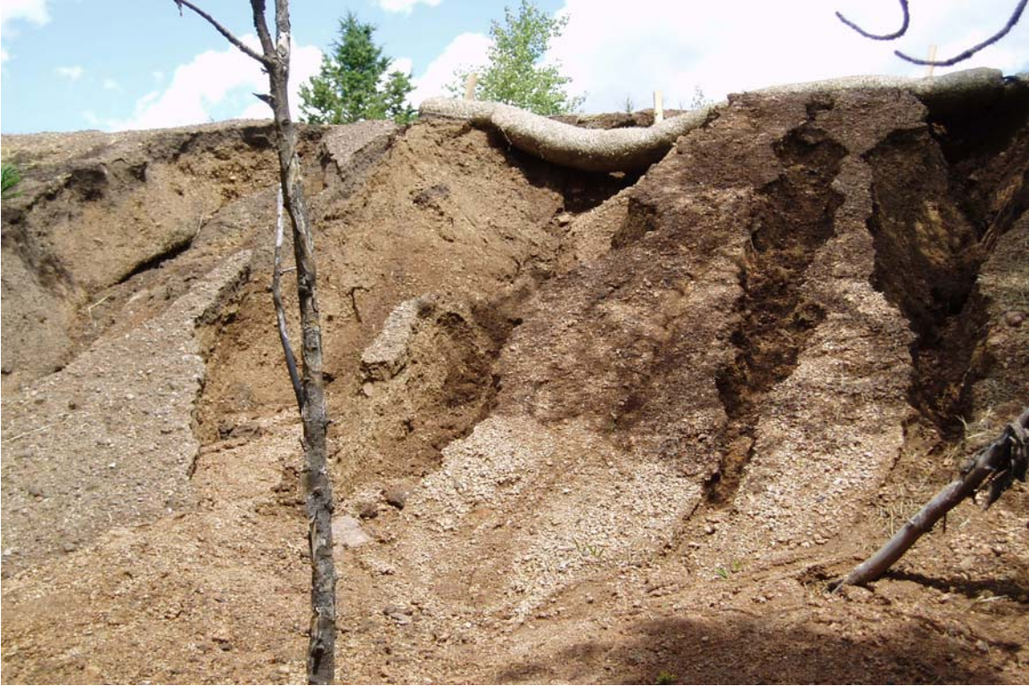
Figure 4. Fill slope failure near 007FS associated with temporary excelsior log control. Note crust of mulch or fiber matrix treatment on slope.
