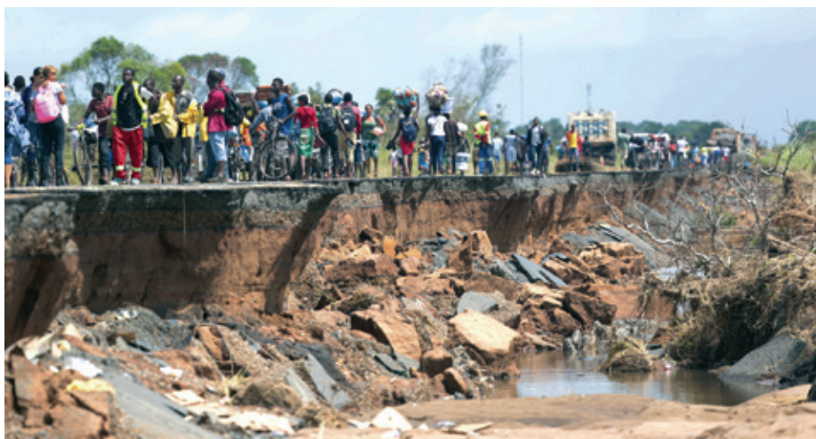
A street destroyed by Cyclone Idai in Nhamatanda, about 50 kilometres from Beira.
