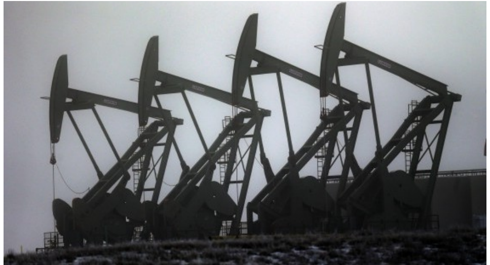
Oil pump jacks work in unison, Williston, USA
