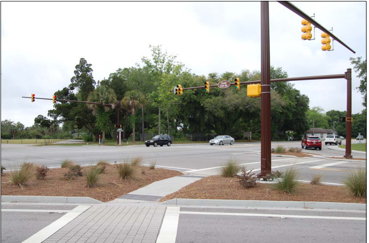
Realignment of the Intersection of US 278 and Squire Pope Road with New Mast Arm Traffic Signals
