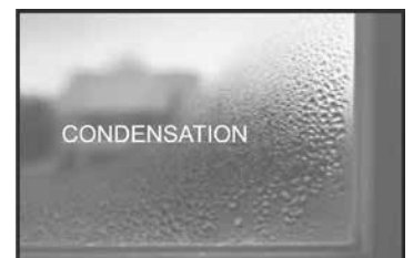
Condensation on a window is an indication of too much humidity.
