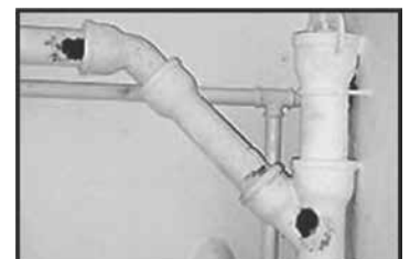
Rust on pipes or other parts of heating, plumbing or air conditioning equipment is also a sign of too much humidity.
