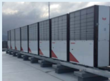
The gas-engine micro cogeneration system introduced at SJR Ropponmatsu
