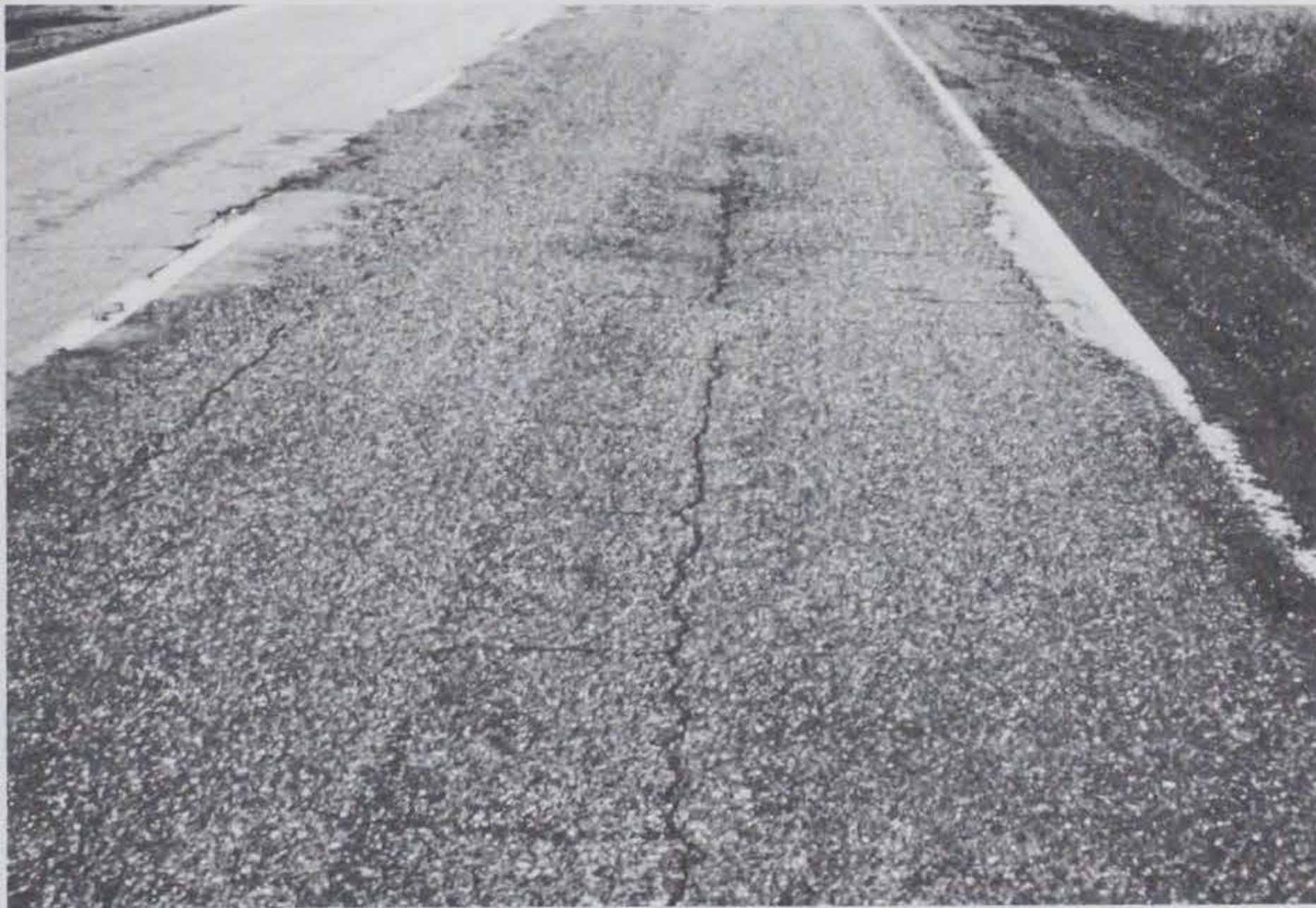
Figure 21. A potential reflective crack
