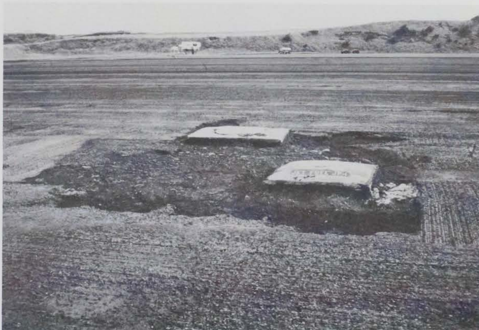
Figure 25. Removal of old pavement and recycling allows the grade of aircraft fueling points on parking apron to be maintained
