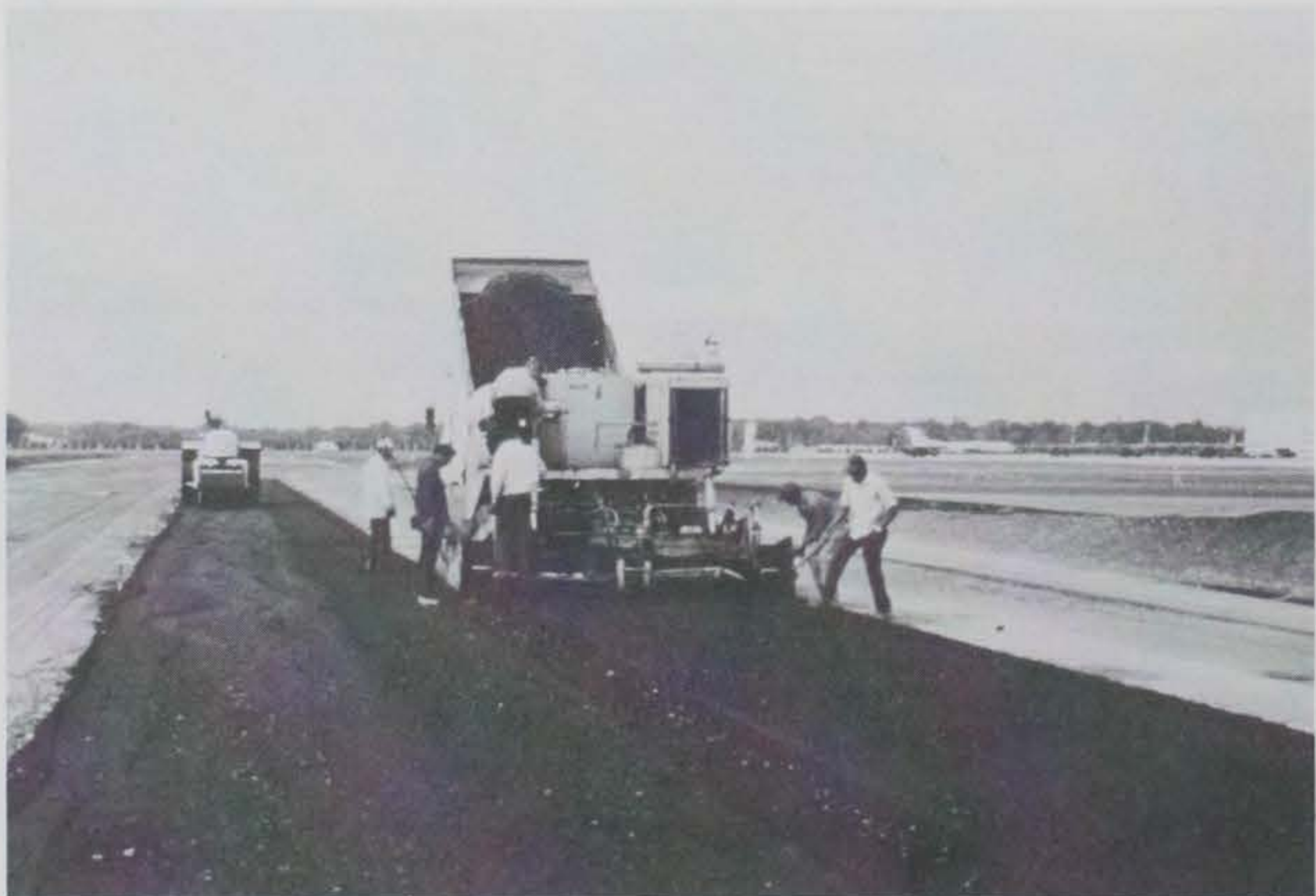
Figure 27. Cold recycling in-place pavement using central plant, then overlaying with conventional hot-mix
