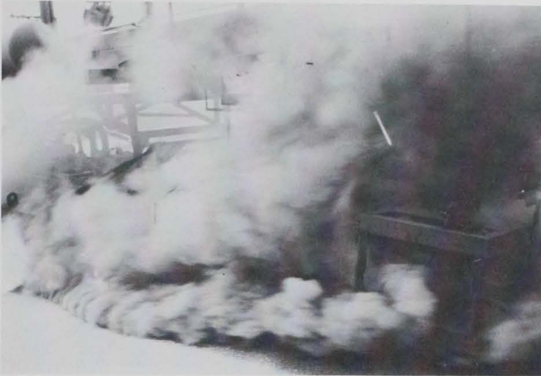
Figure 5. Example of air pollution which can occur during heating of pavement
