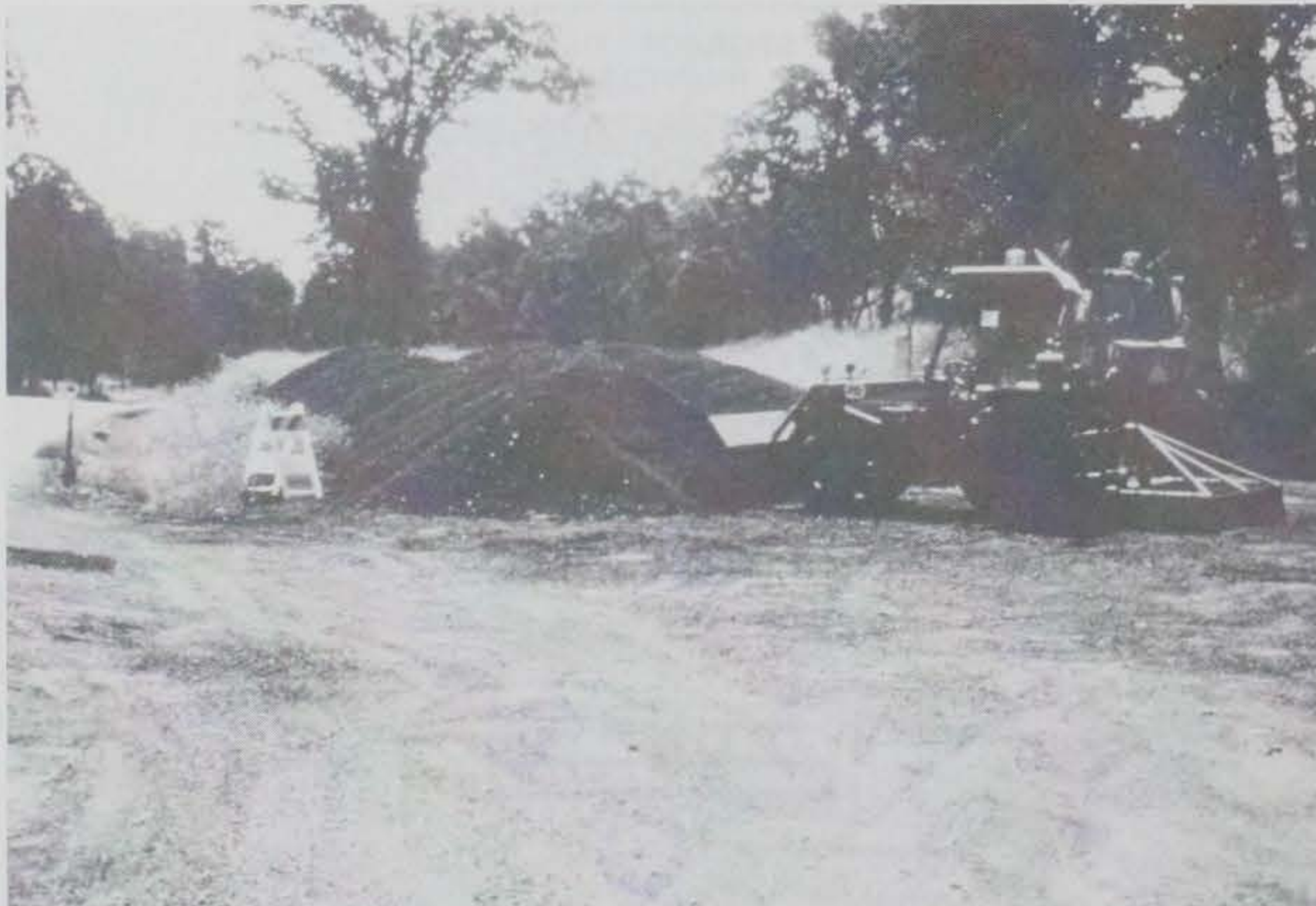
Figure 19. Discarded bituminous pavement
