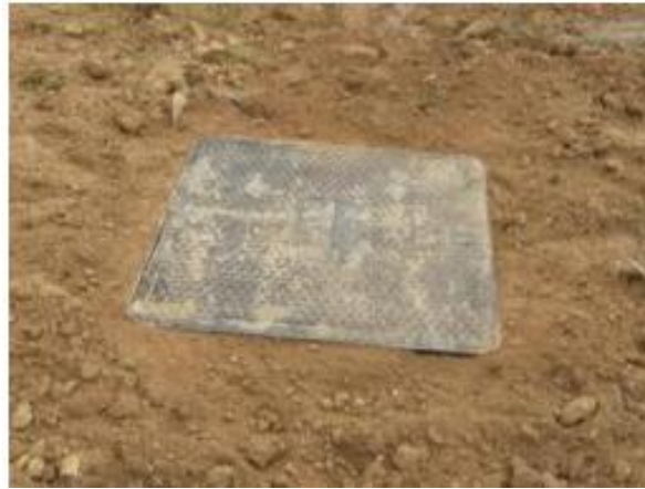
Figure 13. Ground and manhole cover at the same level
